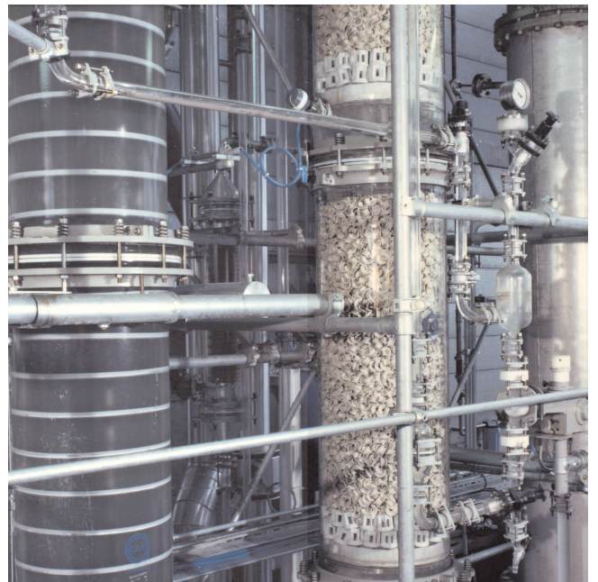
Fig. 1: Sieve plate extraction column and distillation column DN450
